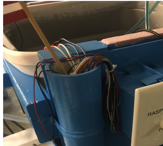
Figure 14. View of finalized Cable Management.
