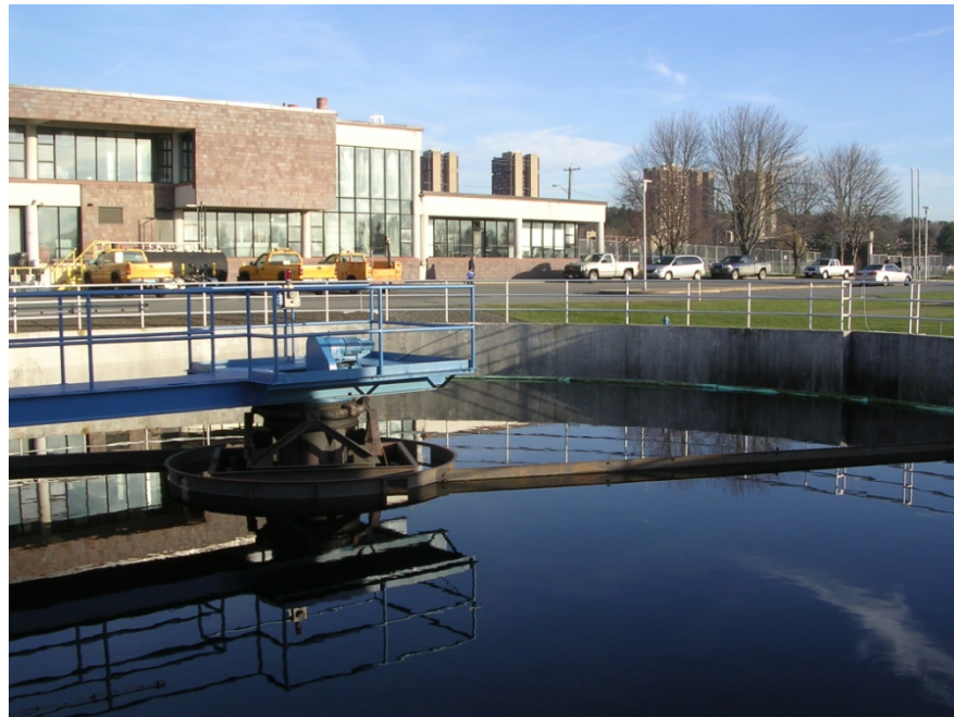
Figure 9. Secondary Clarifier from the Ground
