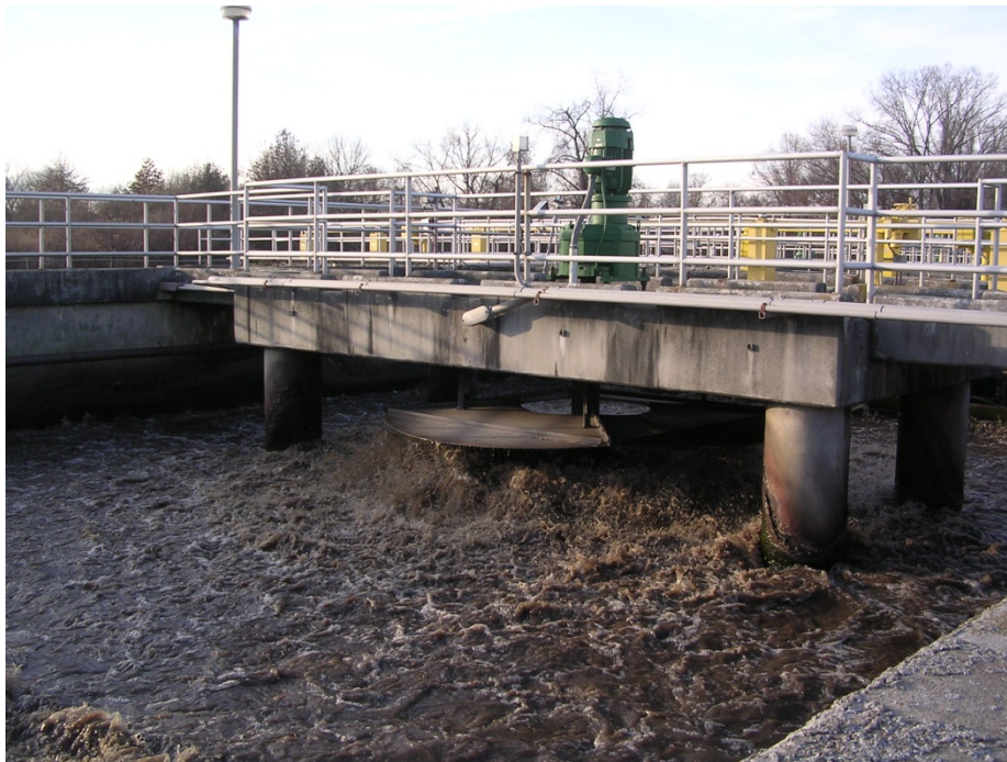
Figure 7. Activated Sludge Tank from the ground showing surface Aerator
