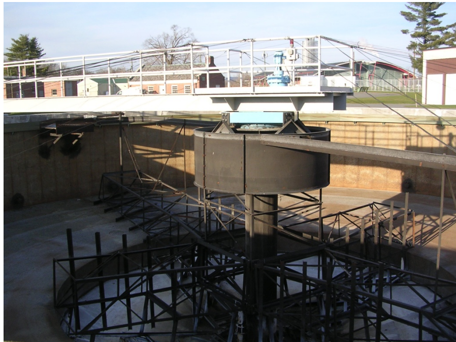
Figure 5. One of the Primary Clarifiers, currently out of Service
